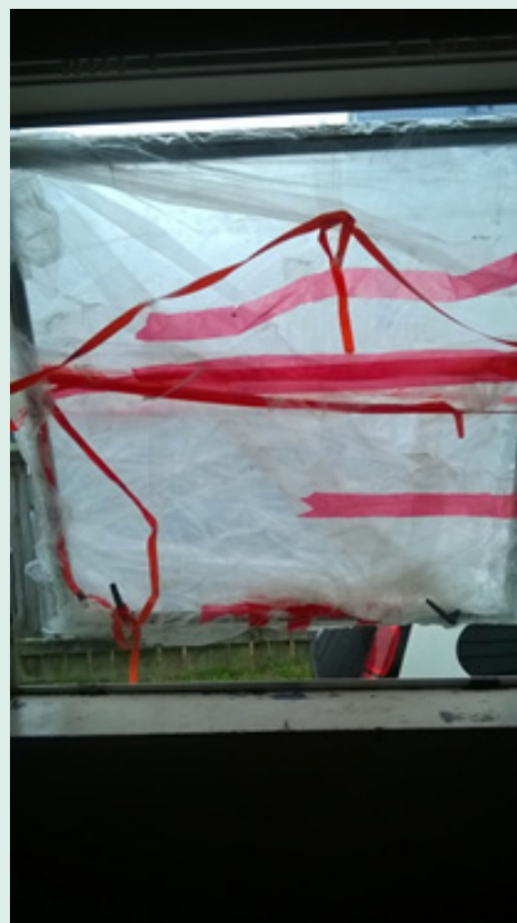
Figure 2. A broken window in a private rental property had been this way for months when the Well Homes assessor visited the house.
